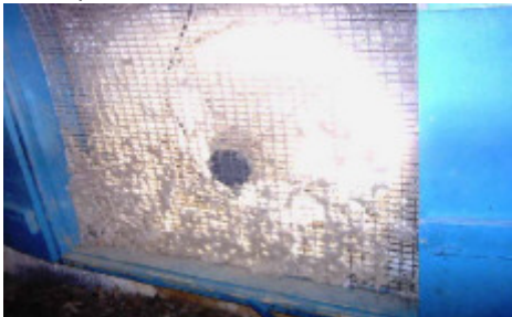
Pic. 3. Dirty bird-protective net resists airflow and strains fan capacity.
